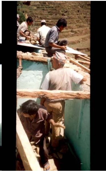
The roof of Future Village was broken by strong wind. Villagers worked together to fix it.
